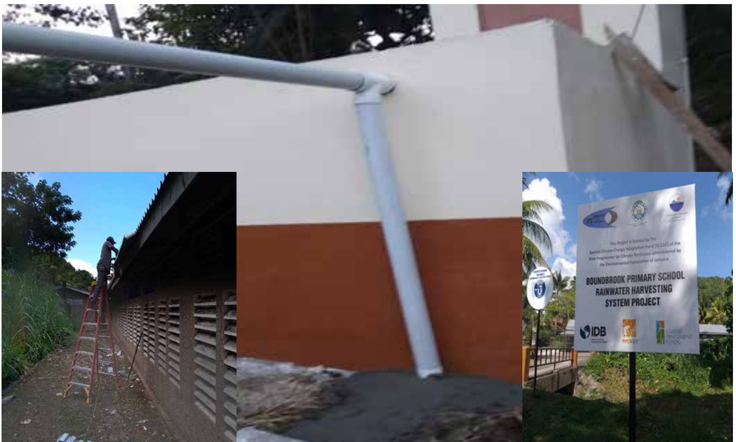
Water Storage tank with conveyance pipes installed. Inset Installation of guttering in progress and erected project sign at entrance of the school
